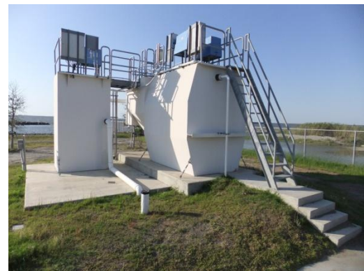
Photo 6 - Flood Protected Pump Station
