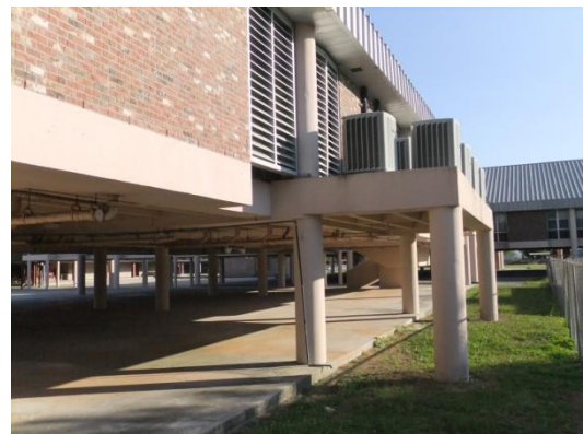
Photo 2 - Flood Protected Mech. Equip.
